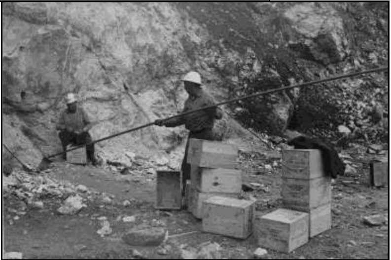
Figure 3: Albert Page loading dynamite into drill holes in the pit wall. (Melvin Mullenix Photograph)
